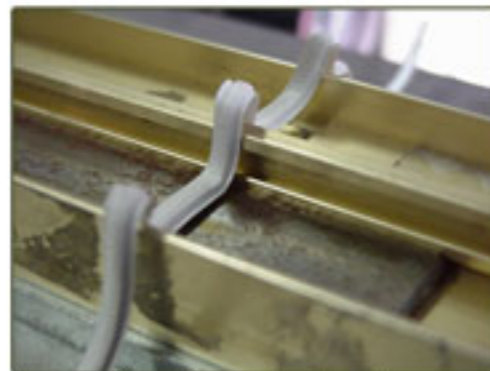
Crushed by window-frame with 2mm. Iron-plate
