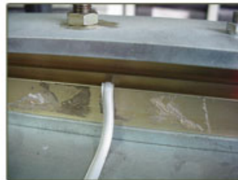
Window closed situation
